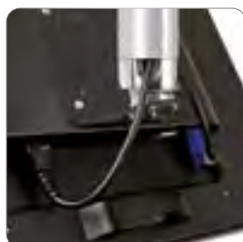
Neatly installed cables
