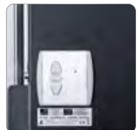
Electric control panel
