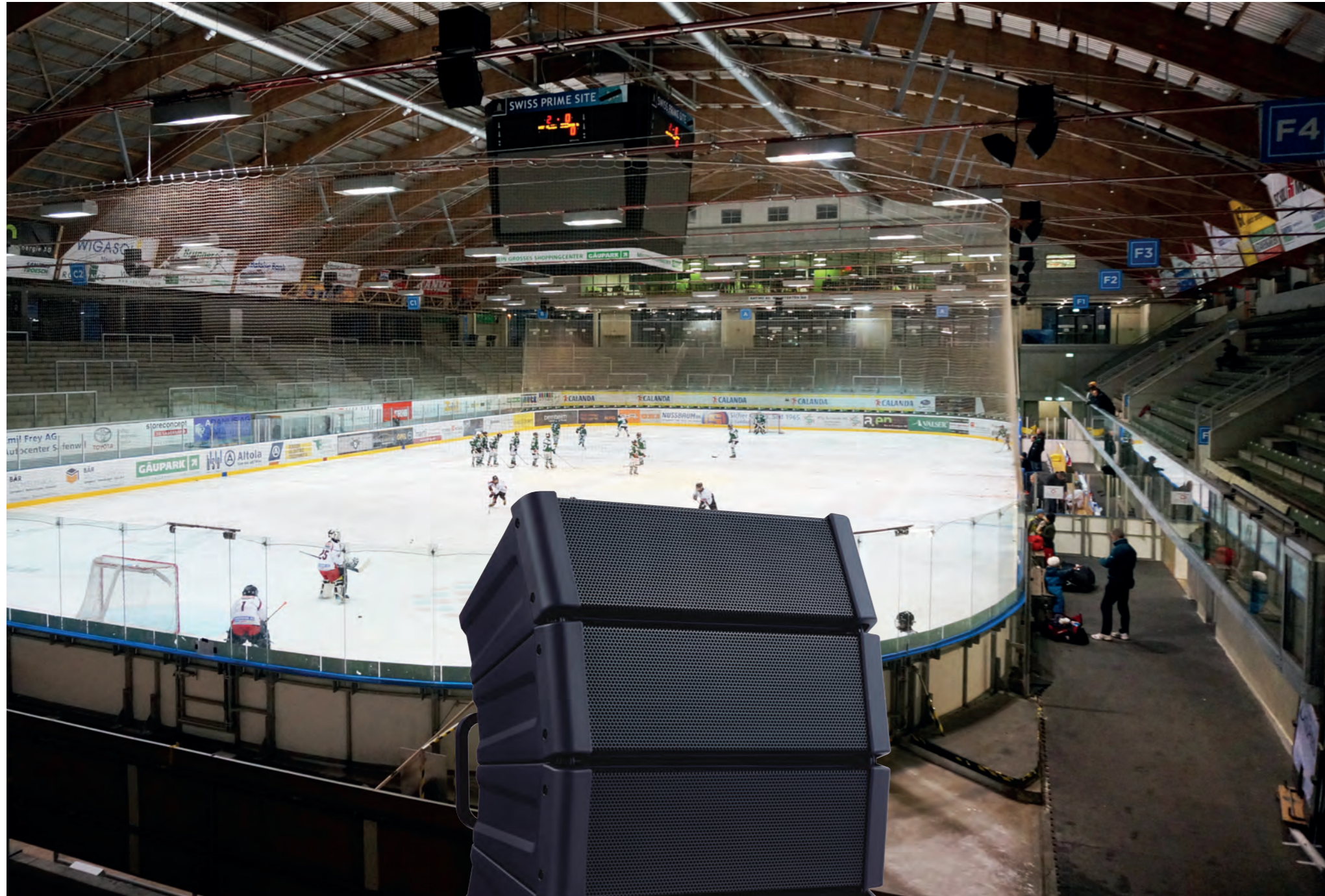
The professional PA in the renovated ice rink in Olten, Switzerland, is realized with Variable Compact Array Speakers HX-5. Low frequencies are supported by FB-120 subwoofers.
