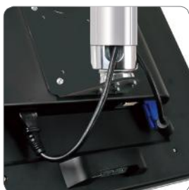
Neatly installed cables
